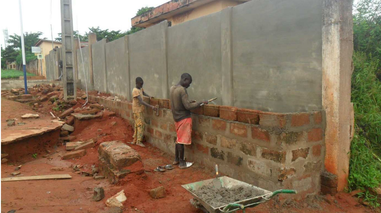
Mason at the service of the ONGED to rebuild the wall of the facade of the CEG1 of Aplahoué
