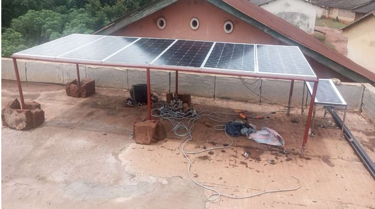
Solar panels for the water tower
